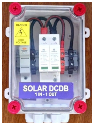
DCDB 1-in/1-out, mounted
